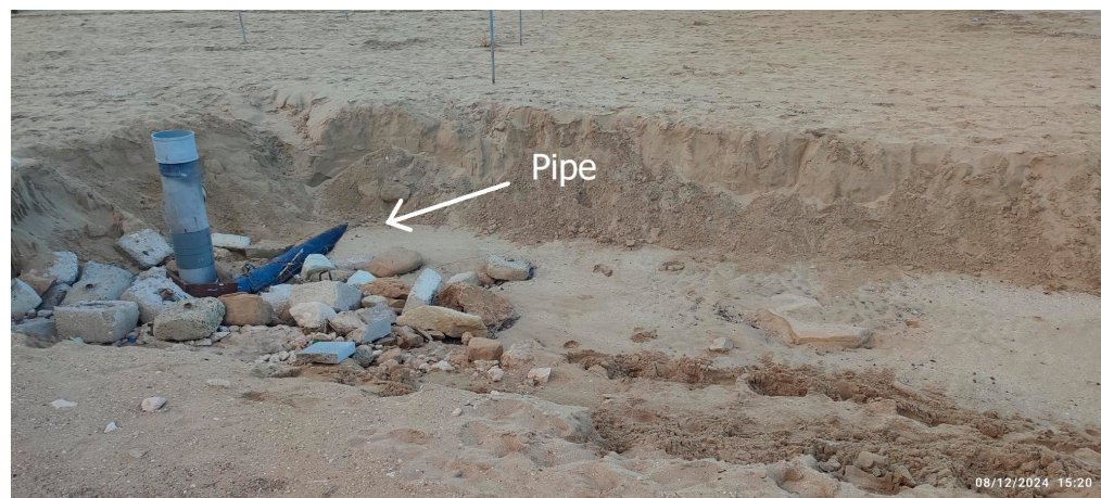
Figure A7. The appearance of a storm drain outlet at the beach surface, as a result of concentrated flow, during the rainy season in grid cell G1 (towards the side of grid cell H2). The image was captured on 8 December 2025 at 03:20 p.m.
