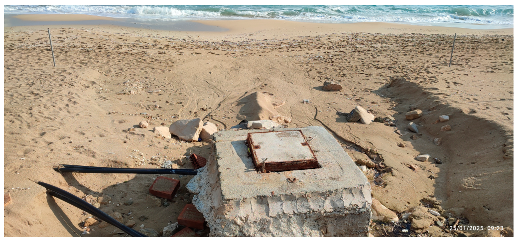
Figure A6. Exposed stormwater drainage infrastructure in grid cell I2. The image was captured on 25 January 2025 at 09:23 a.m.
