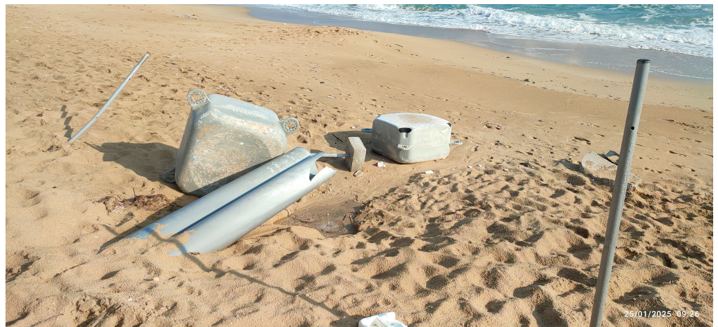
Figure A5. Exposed stormwater drainage infrastructure in grid cell G1. The image was captured on 25 January 2025 at 09:26 a.m.
