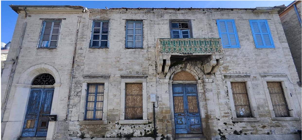
Figure 1 Listed building located in Limassol's historic district with visible damage patterns due to thermal stress.
