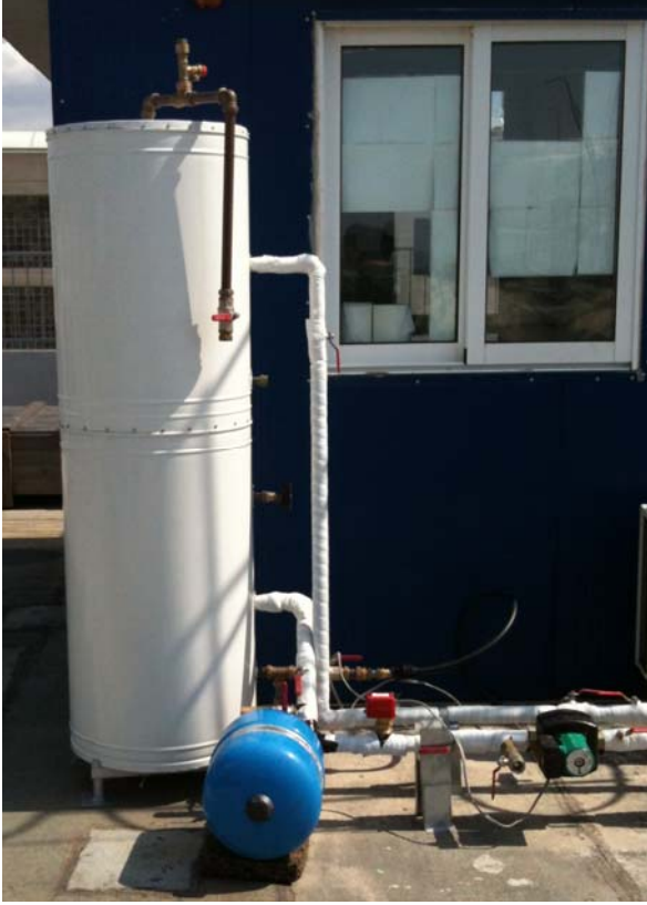
Fig. 5: Photo of the storage tank
