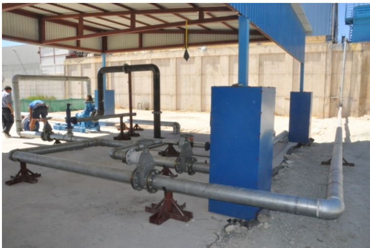
Figure 7. Photo of a part of the pipe network as it has been constructed
