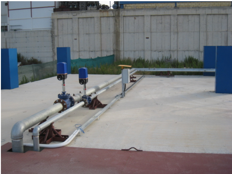
Figure 15. Long straight pipe segments where the friction losses as measured.
