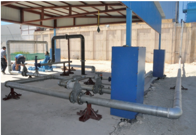
Figure 7. Photo of a part of the pipe network as it has been constructed
