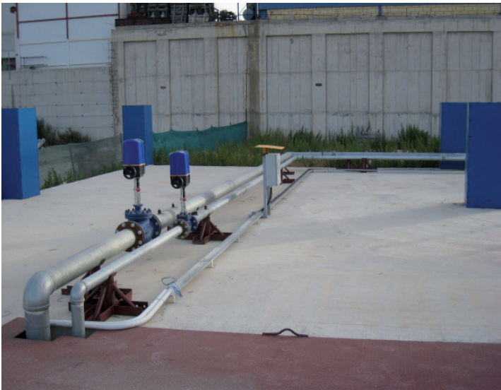
Figure 15. Long straight pipe segments where the friction losses as measured.
