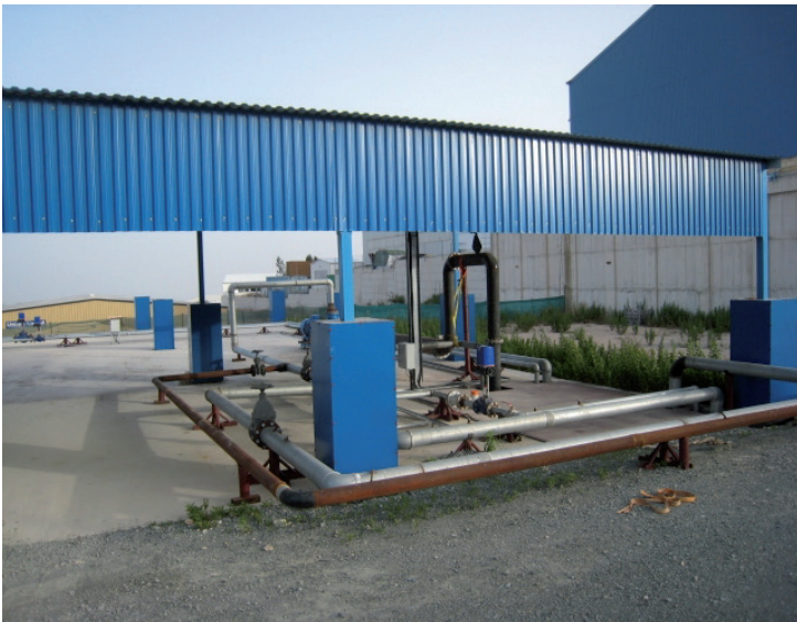
Figure 13. Overview of the pipe network
