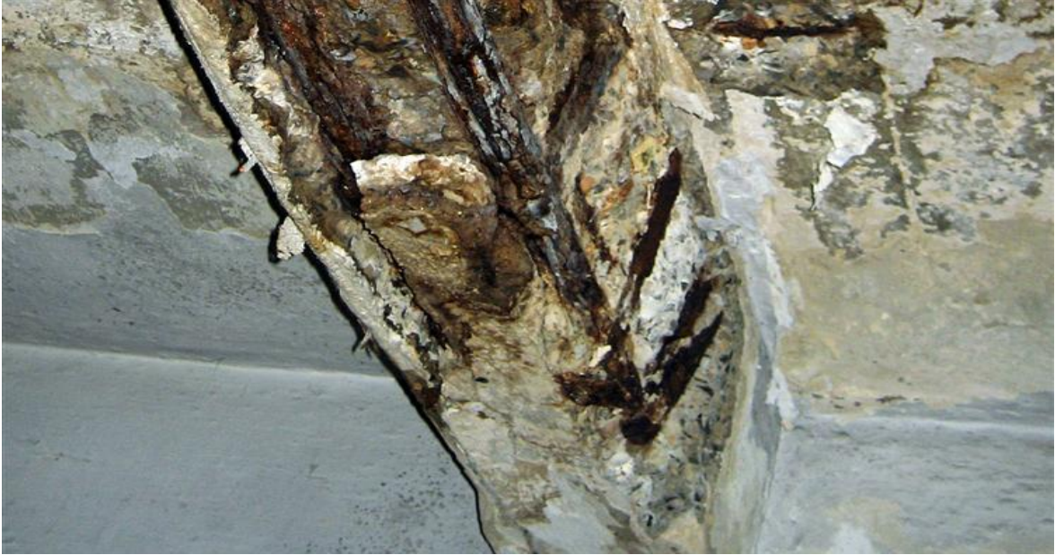
Figure 8: Severe corrosion condition of a column
