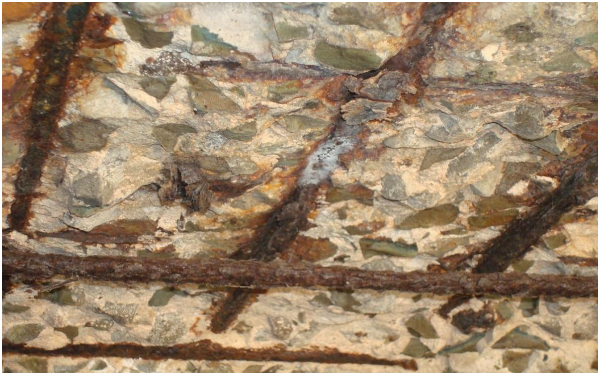
Figure 5: Corroded steel of a slab and delamination of concrete cover
