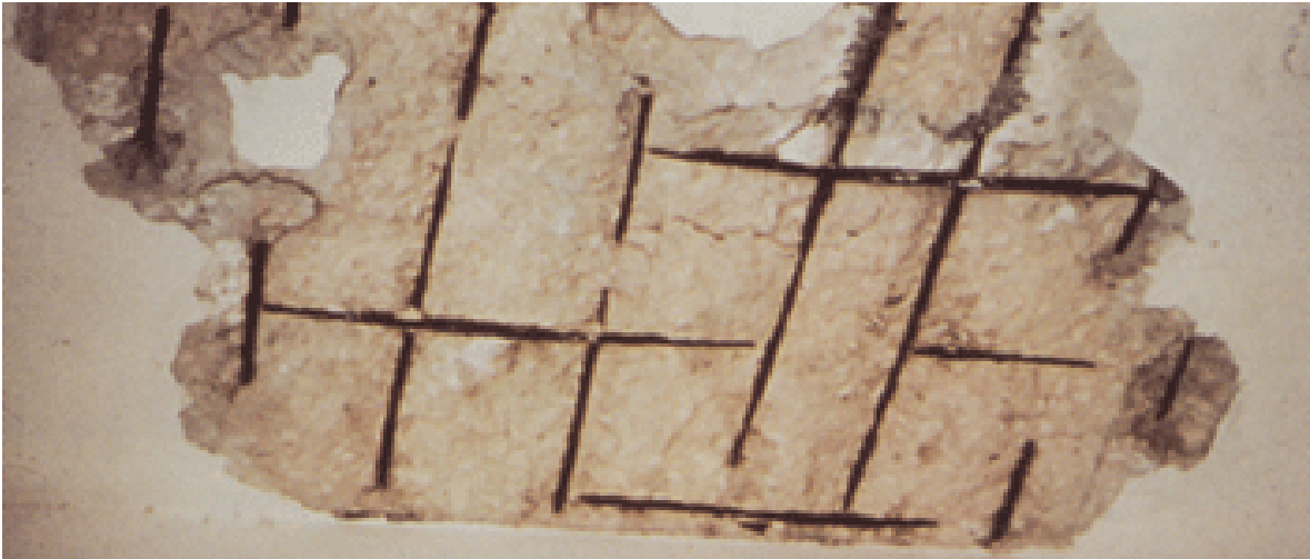
Figure 6: Corroded steel and delamination of the cover layer on a basement
