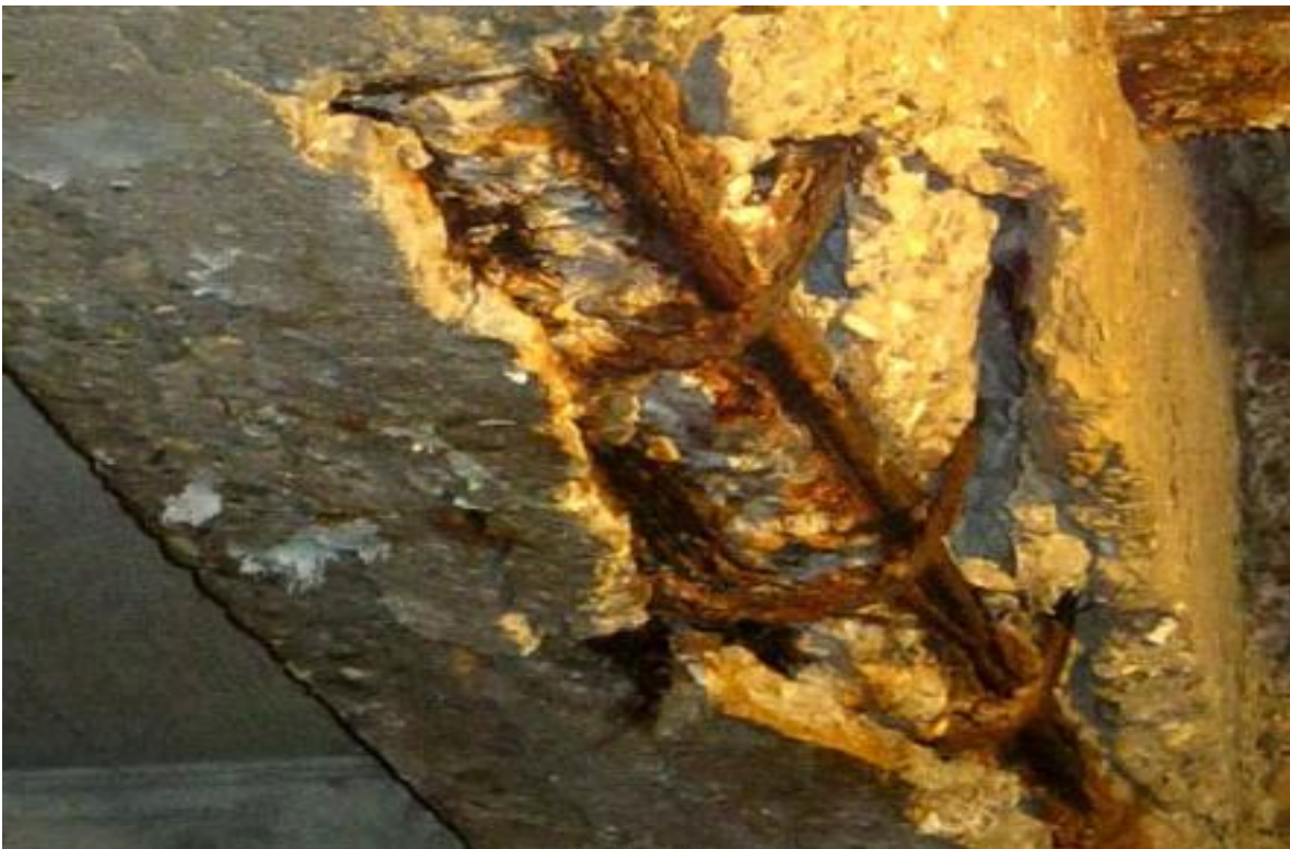
Figure 7: Corrosion of the whole system of reinforcing bars (longitudinal and stirrups) on a concrete beam
