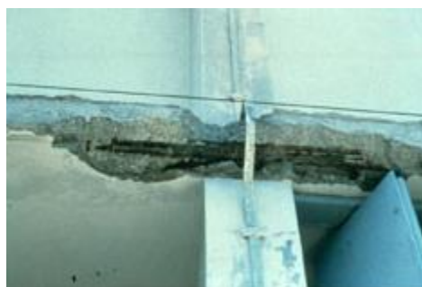
Figure 11: Example of carbonation (“Corrosion of Embedded Materials” n.d.)
