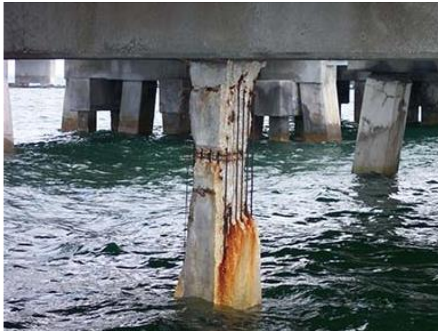
Figure 12: Corrosion due chlorides in seawater (“New methodology predicts onset, progression of corrosion of reinforced concrete” n.d.)
