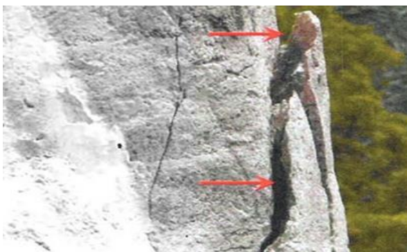
Figure 1: Delamination of concrete (“Funds needed for Black Hawk Statue restorationThe Rock River Times | The Rock River Times” n.d.)
