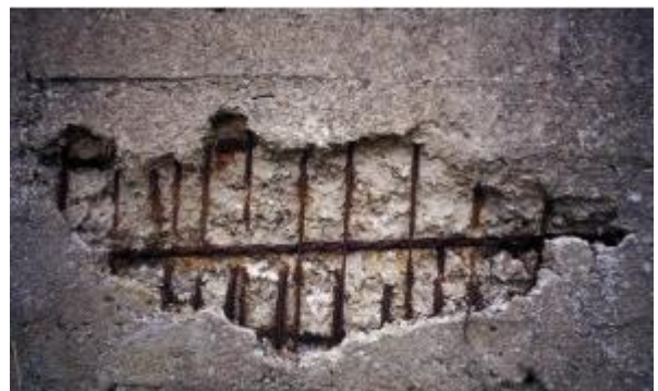
Figure 2: Spalling of the concrete (“Spalling of Concrete - Causes, Prevention & Repair - CivilDigital - Anand Paul” n.d.)
