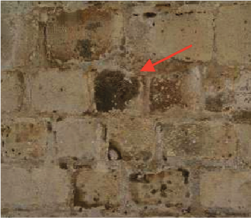
Figure 17: Incrustation on the surface of limestone block.
