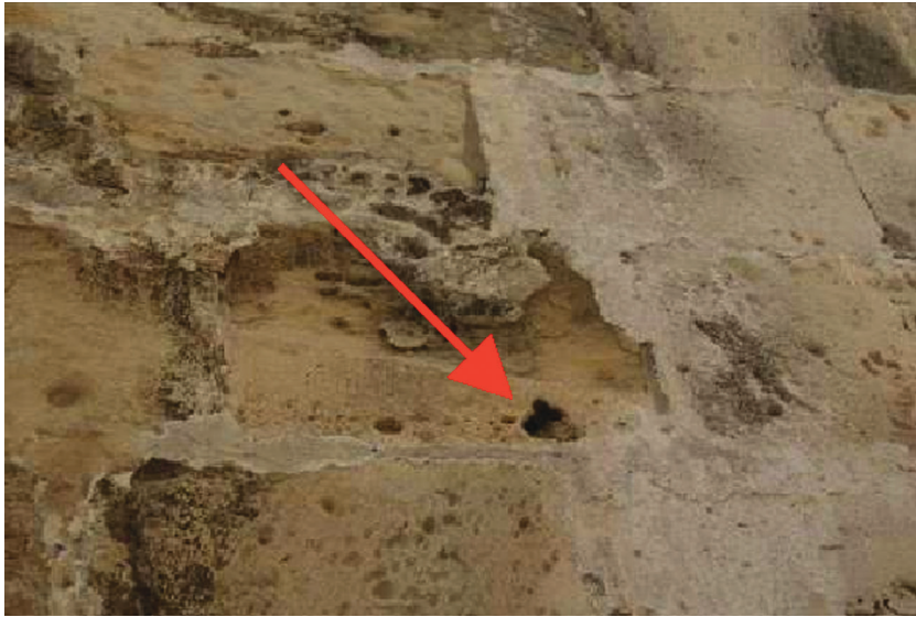
Figure 19: Physical loss of material from the surface of the block.
