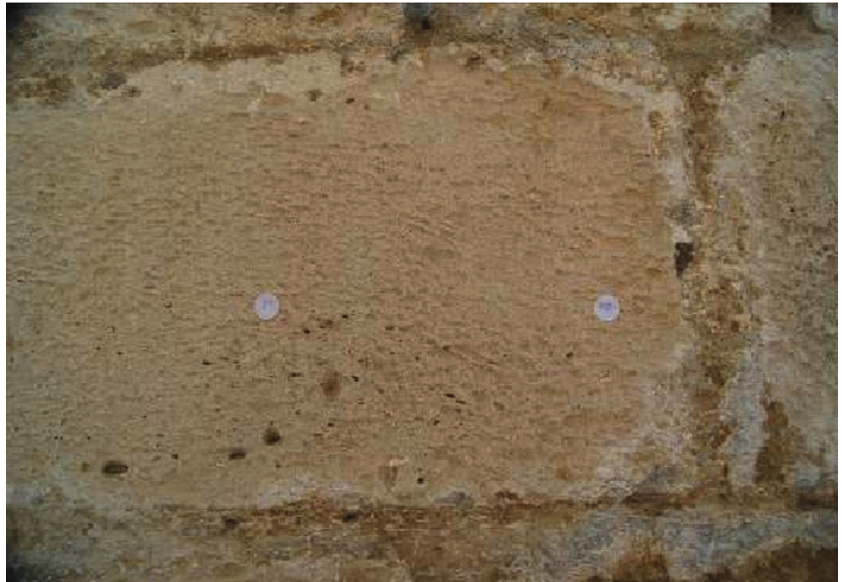
Figure 21: Acupuncture like corrosion on the surface of limestone block.
