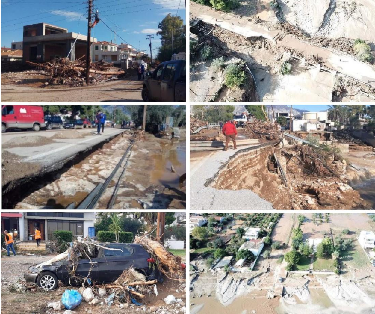
Figure 3: Damages by the flood of 2019 to infrastructure, road networks, and the coastline of the Kineta area [111,114,115].
