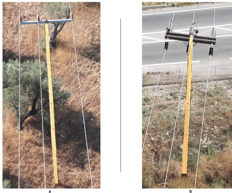
Figure 8. (a,b) Tilted electric poles of the investigated power network on Lesvos Island.
