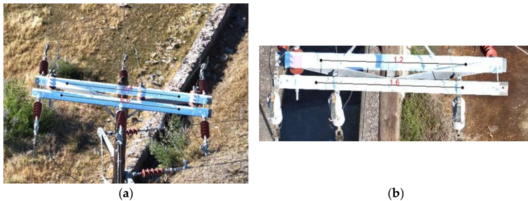
Figure 9. (a,b) Tilted crossarms observed in the under-study network.
