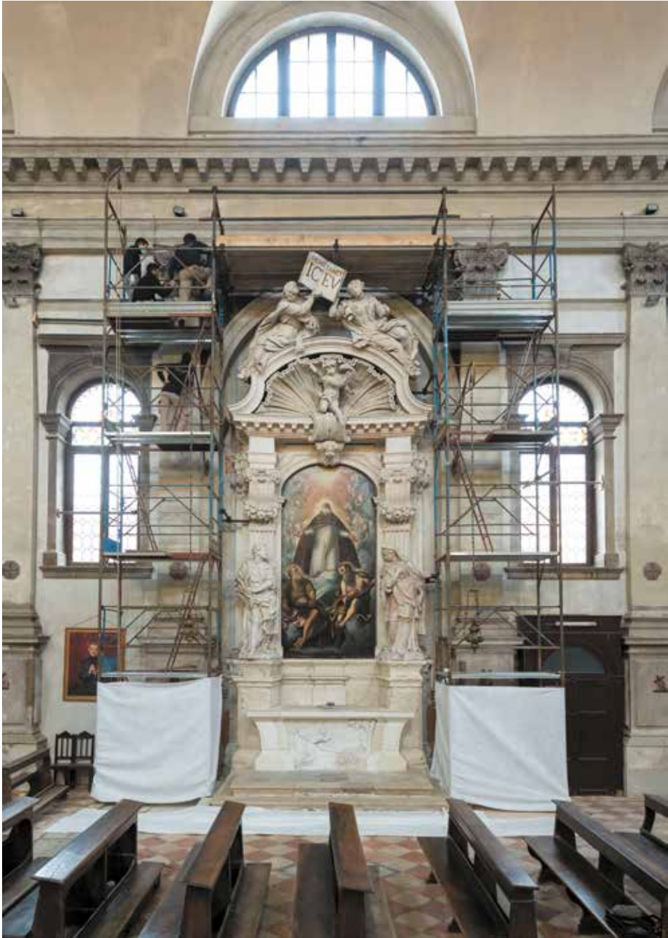
Figure 10.3 Scaffolding set up for the 2022 de-installation of the St Luke and St John spandrels above the altar of St Martial with its altarpiece by Jacopo Tintoretto (1549), San Marziale, Venice. Photograph by Matteo De Fina, courtesy of Save Venice.
