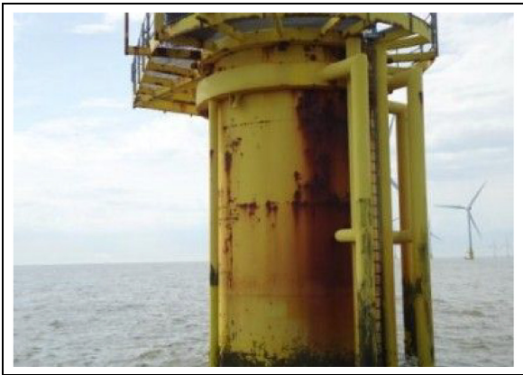
Figure 8. Extents of corrosion in a monopile of an OWT. 54
