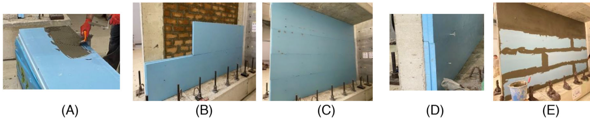
FIGURE 6 XPS boards application steps (A) adhesive material at the surface of the XPS using notched trowel, (B) application of the first and second strips of XPS board, (C) infilled frame with four and half XPS boards, (D) application of special plastic dowels, and (E) adhesive material at the surface of the XPS using notched trowel.
