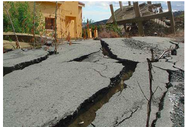
Figure 2. Landslide effects in Pissouri area
