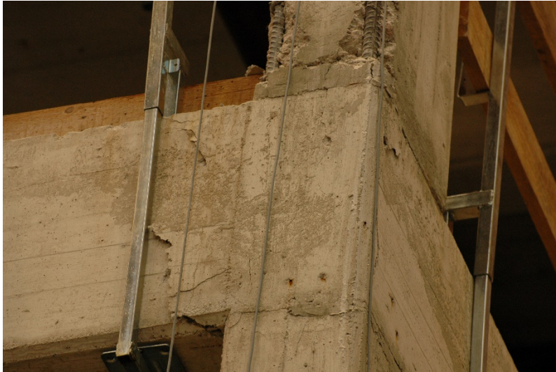
Figure 8.14 Position 29: Cracks propagated into the cross beam
