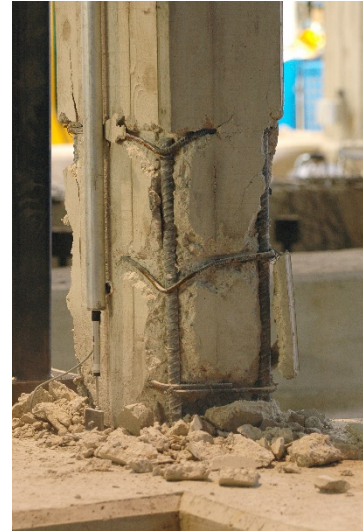
Figure 8.15 Position 8: Column is severely damaged
