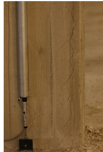
Figure 8.11 Position 1: Damage to the north wall column
