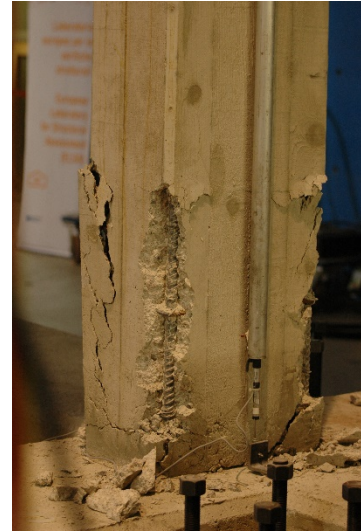
Figure 8.3 Position 8: Failure of the column at the bottom
