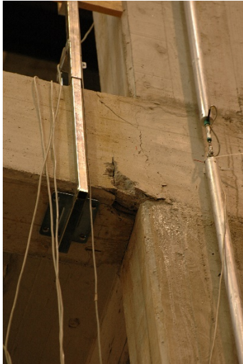
Figure 8.8 Position 30: Beam next to the wall is cracked
