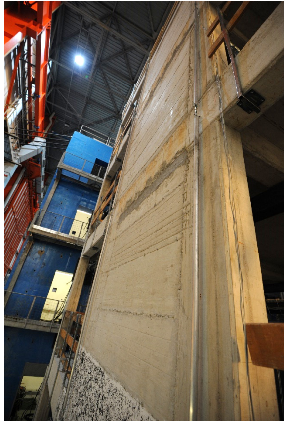
Figure 6.7 Instrumentation on the outside face of the central bay, north frame
