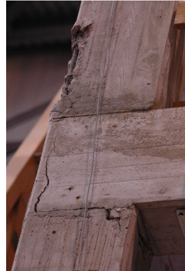
Figure 8.7 Position 29: Failure of the lap splice joint, S frame
