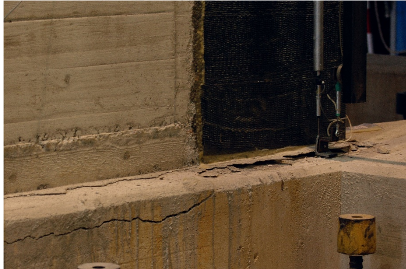
Figure 8.9 Position 7: Horizontal crack developed also in the foundation beam
