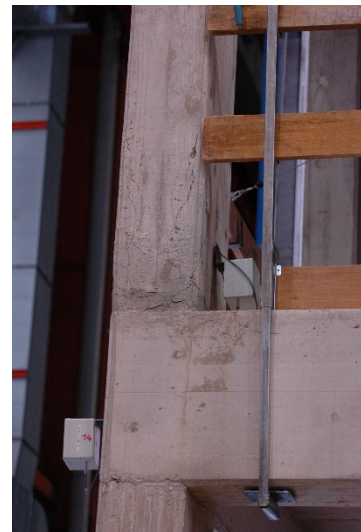
Figure 8.5 Position 12: Failure of the laps splice joint, N frame
