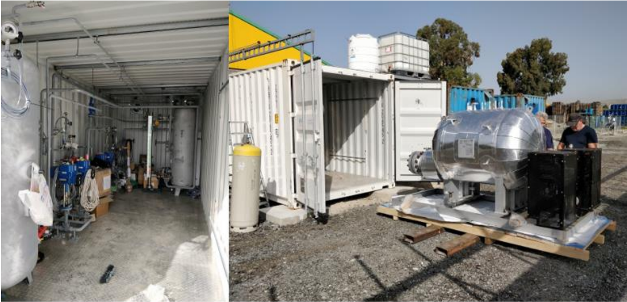
Figure 92: Steam Generator shipped and ready to be installed.
