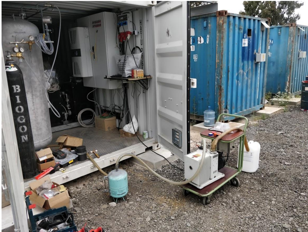
Figure 94: System filled up with HTF and the expansion tank with nitrogen.
