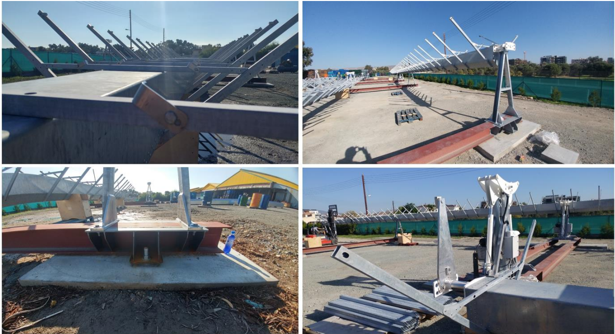
Figure 83: Mirror, absorber tube basis, and setting the PTC on the structure.
