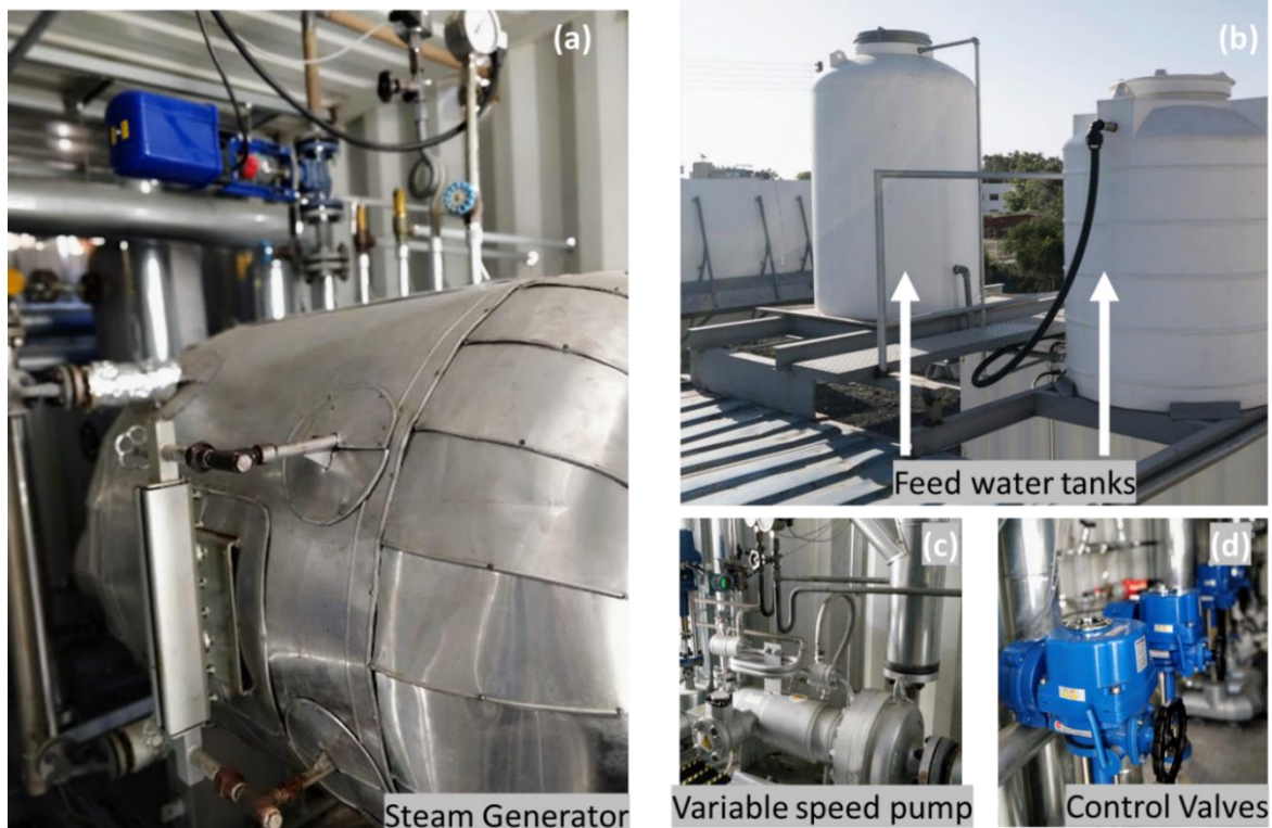
Figure 49: (a) SG (b) Feed water tank (c)Variable speed pump (d) Control valves.
