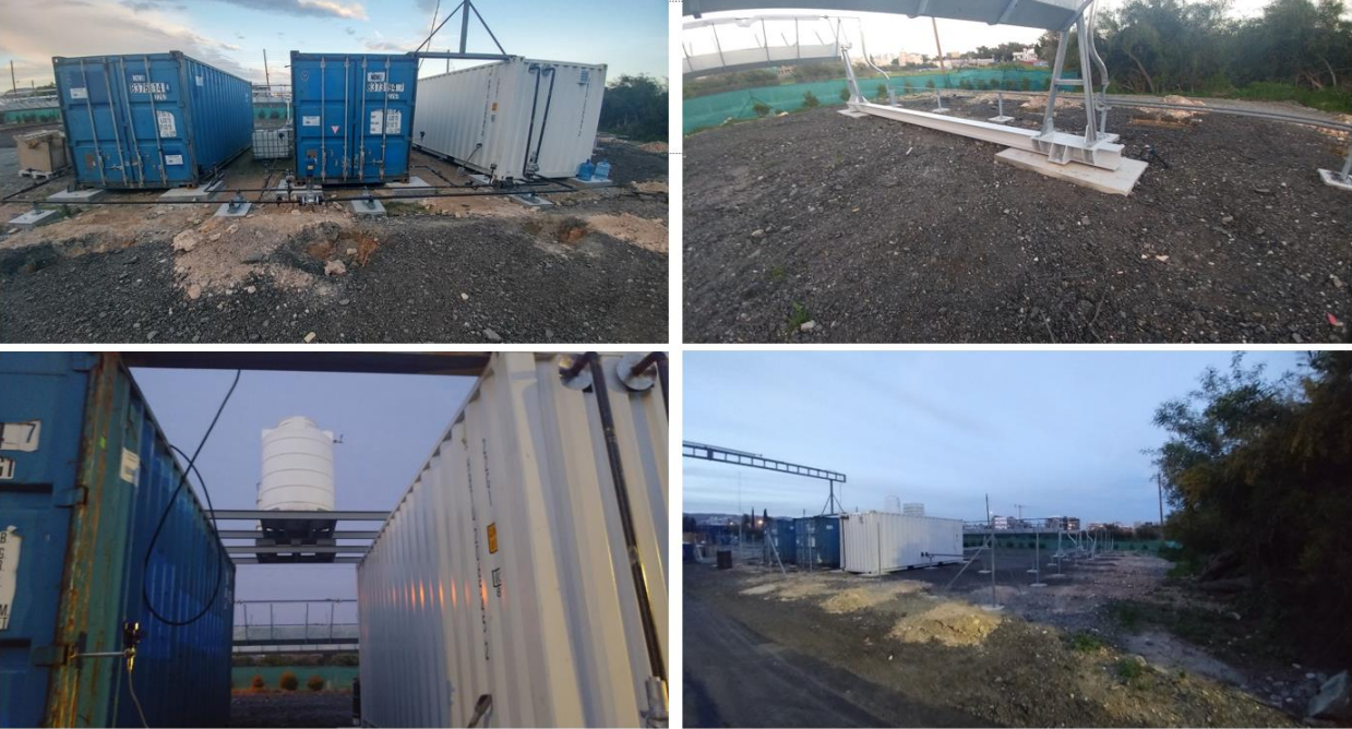
Figure 90: Painting the containers and other equipment, and the installation of the feed water tank.
