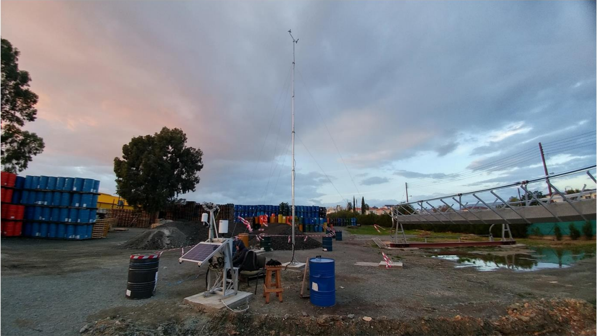
Figure 91: Installation of the weather station.
