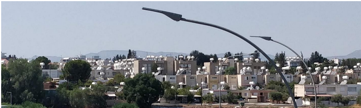
Figure 29: Thermosyphon solar water heating type installed on the roof of the domestic sector and tourist apartments.
