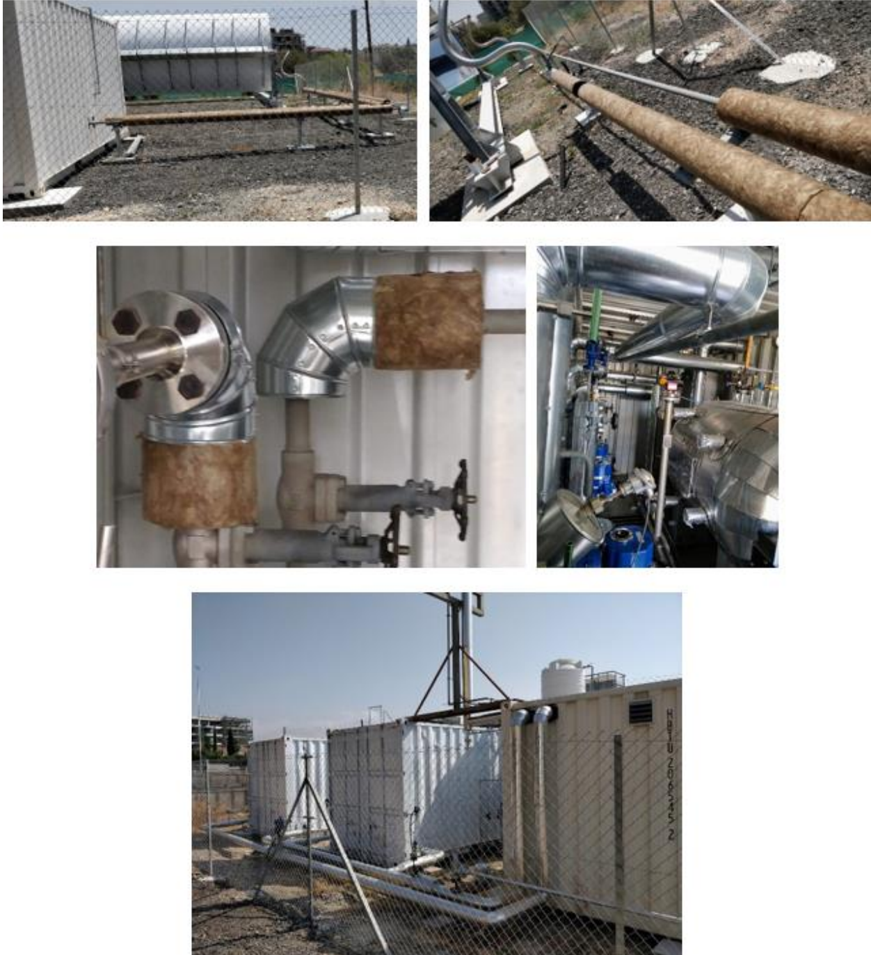
Figure 98: Thermal insulation on various parts of the system.
