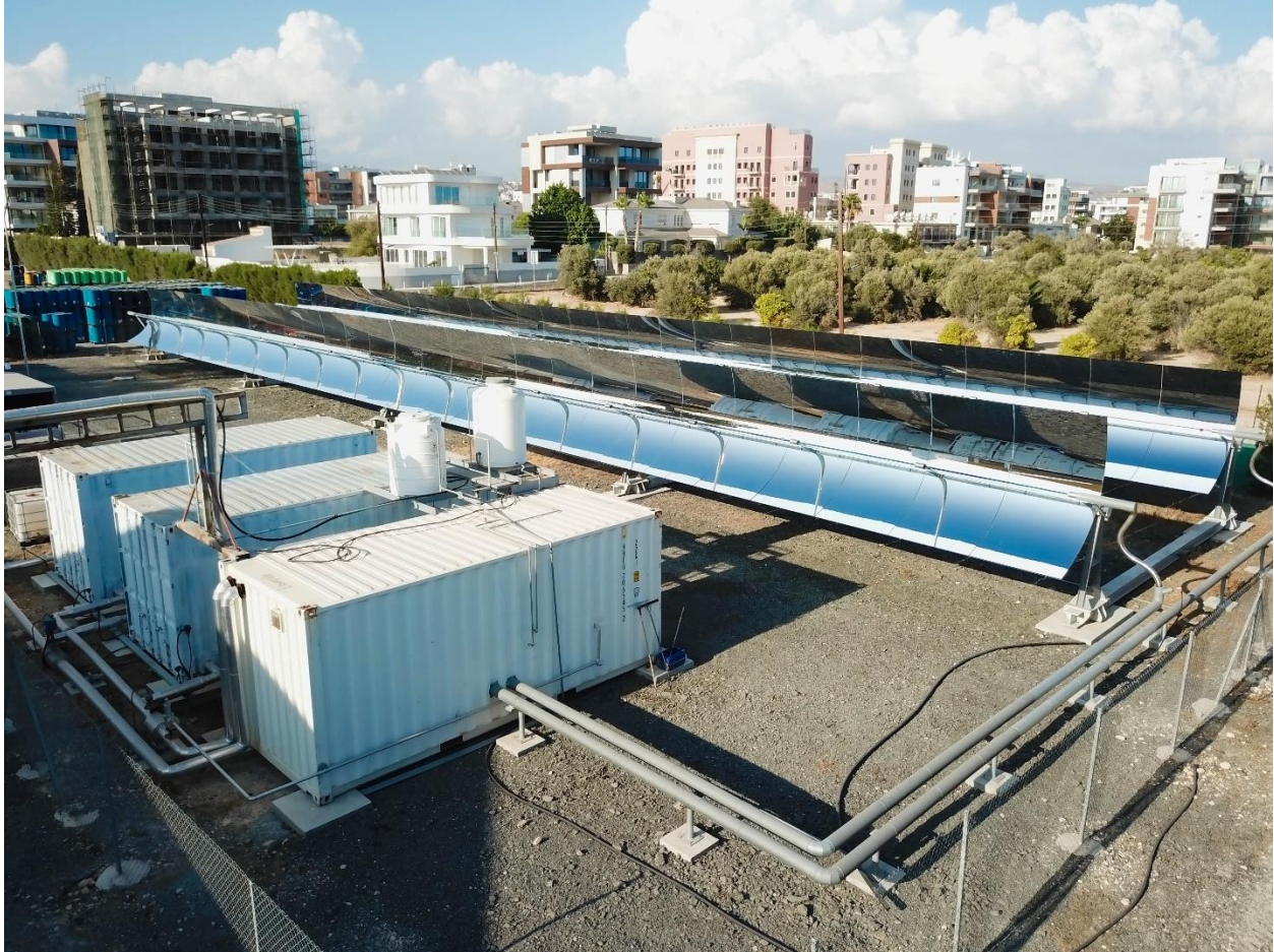
Figure 46: PTC system installed and operating.
