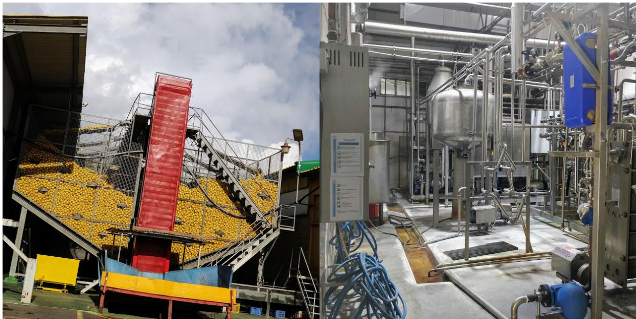
Figure 44: Process in Kean factory which requires thermal energy.
