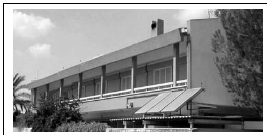
(b) Installation detached from the house
