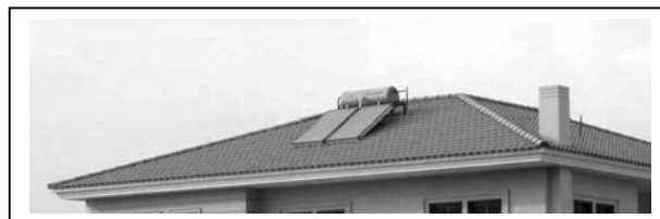
Fig. 3 Pressurised solar water heater installed on an inclined roof.
