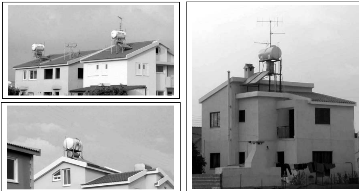
Fig. 3 Applications of tower-type solar water heaters installed on inclined concrete roofs.
