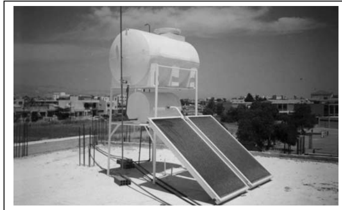
Fig. 2 Typical application of tower-type solar water heater installed on flat roof.
