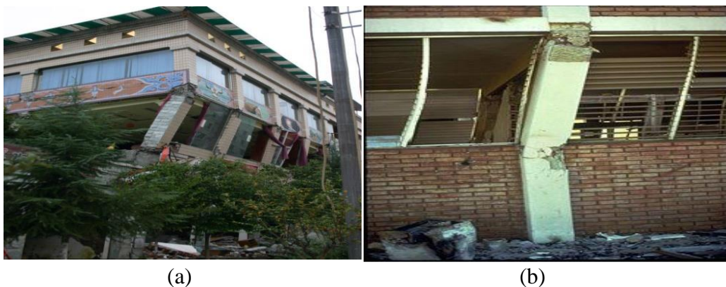
Figure 2.1: Typical failure mechanisms of masonry-infilled RC frame buildings: (a) soft-story mechanism (Çağatay 2005) and (b) short-column mechanism (Pradhan et al. 2012).
