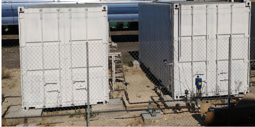
FIGURE 4. C-TES modules in containers at the KEAN factory in Limassol, Cyprus
