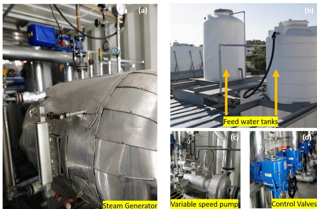
Fig. 5. (a) Steam generator (b) feed water tanks (c) variable speed pump (d) control valves. The authors would like to apologise for any inconvenience caused.
