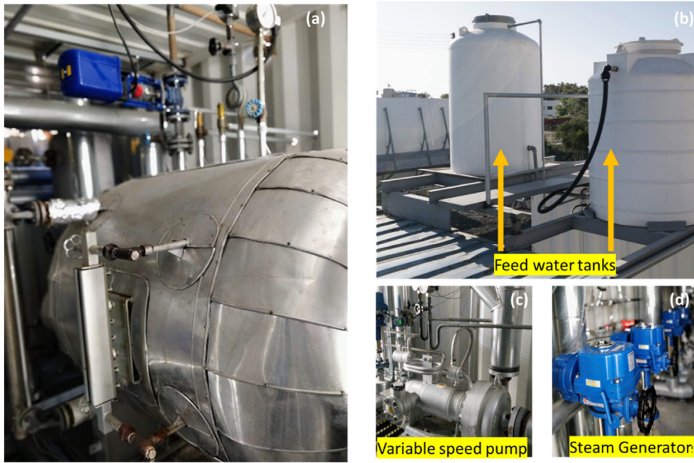
Fig. 5. (a) Feed water tanks (b) variable speed pump (c) control valves (d) steam generator.
