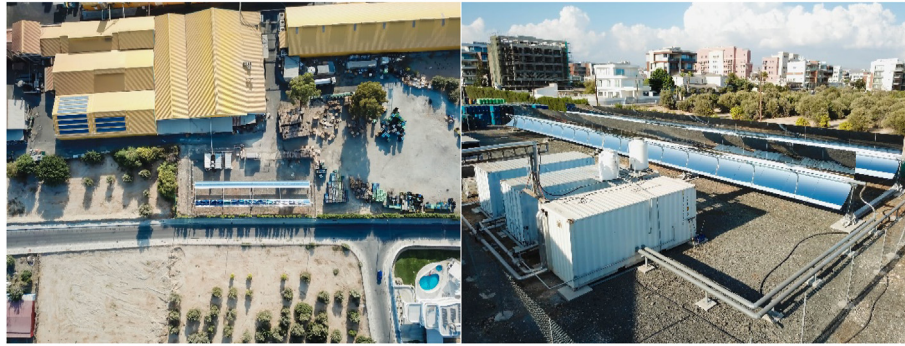
Fig. 2. Sky-view showing the KEAN factory and the location of the PTC system (left) and the PTC system in a closer view (right).
