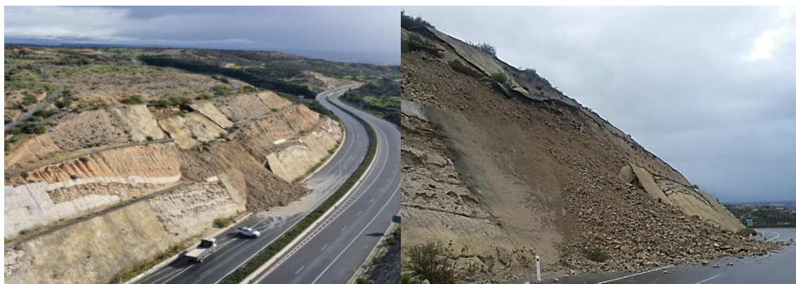
Figure 85: Landslide near Pissouri by the A6 motorway (Geological Survey Department)
