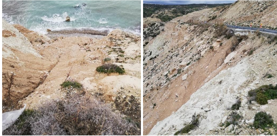
Figure 30: Landslide near Paphos-Limassol old road next to Petra tou Romiou (source: Geological Survey Department)
