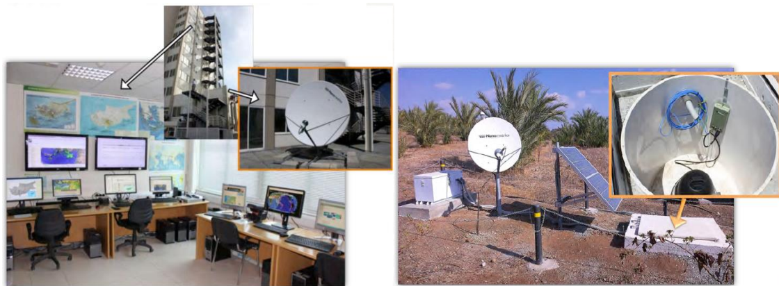
Figure 13: The primary seismological centre (left) and the prototype seismological station GSD in Nicosia (right) (source: Geological Survey Department)
