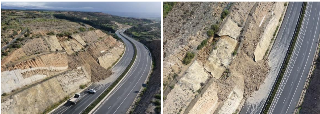
Figure 29: Landslide on the Paphos-Limassol motorway near Pissouri (source: Geological Survey Department)
