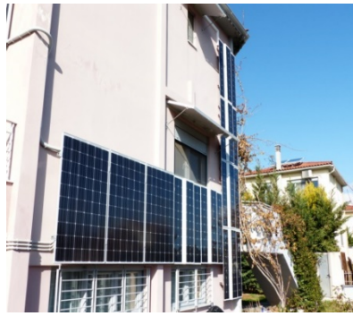
Fig. 2 Facade PV Subsystem
