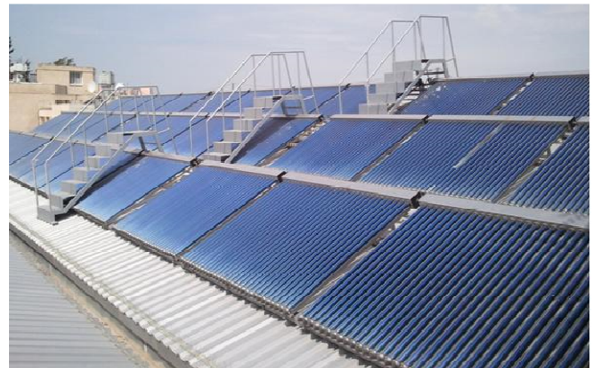
Fig. 3 Photo of one of the two banks of solar evacuated tube collectors
