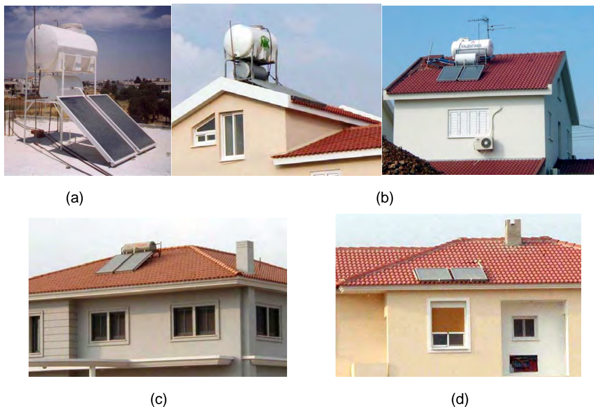
Fig. 1: Various flat-plate solar water heating systems in Cyprus (a) Typical flat roof; (b) Installation on sloping roof to improve aesthetic appearance; (c) Pressurized system on sloping roof; (d) Forced circulation system on flat roof
