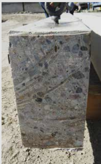
Figure 3. Extreme abrasions due to saw cutting on beam end.
