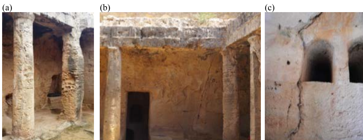
Figure 9. Pilasters and columns at the atrium of the tomb that exhibit cracking and fracturing at the base (a) and fissures at the exterior (b) and interior (c) of the chamber compartment.
