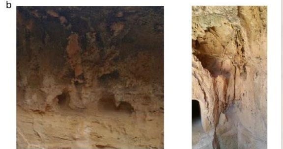
Images from: Kyriakides et al. (2016), Correlating damage condition with historical seismic activity in underground sepulchral monuments of Cyprus, Journal of Archaeological Science: Reports
