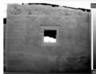
GPR, Sonic and (in case) infrared thermography data integration for the dection of buiding and decay features
