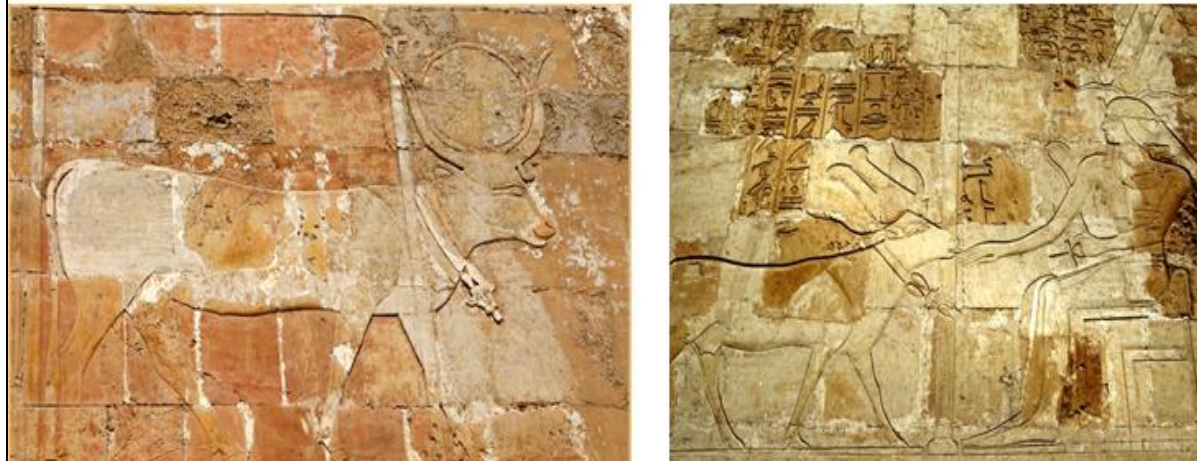
Deterioration in the walls of Hatshepsut temple
