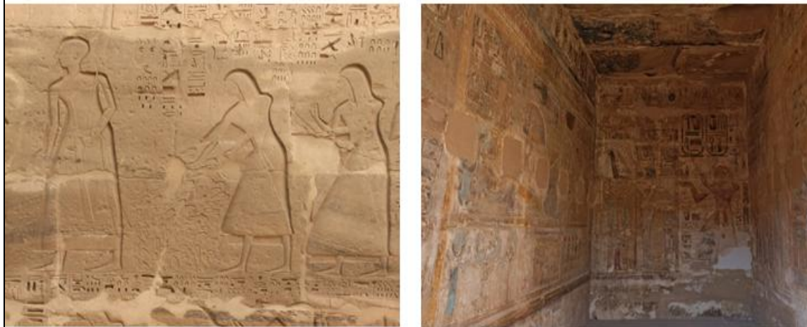
Deterioration in the walls of Medinet Habu temple ( http://www.touregypt.net/featurestories/waterdamage.htm )
