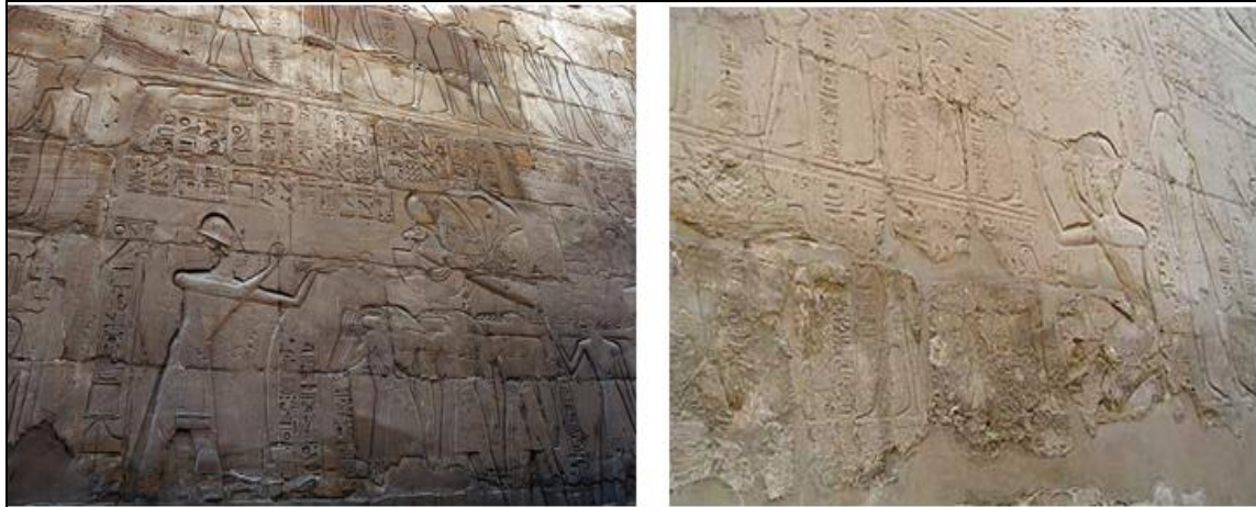
Deterioration in the walls of El Karnak temple ( http://www.touregypt.net/featurestories/waterdamage.htm )
