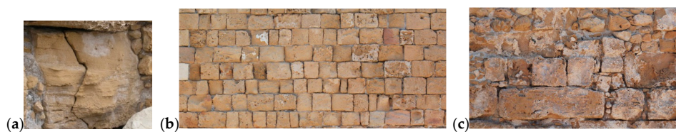
Figure 4. Individual fissures, clearly visible to the naked eye (a); Loss of mortar joints between the masonry blocks (b); Surface discoloration in the form of salt efflorescence pattern (c).
