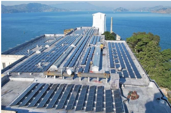
Figure 1.2. Photovoltaic panels on the roof of a building.
