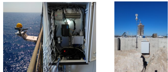
Figure 1 Monitoring system in Vasiliko VTTV (left) and Ayia Napa Marina (right), Cyprus
