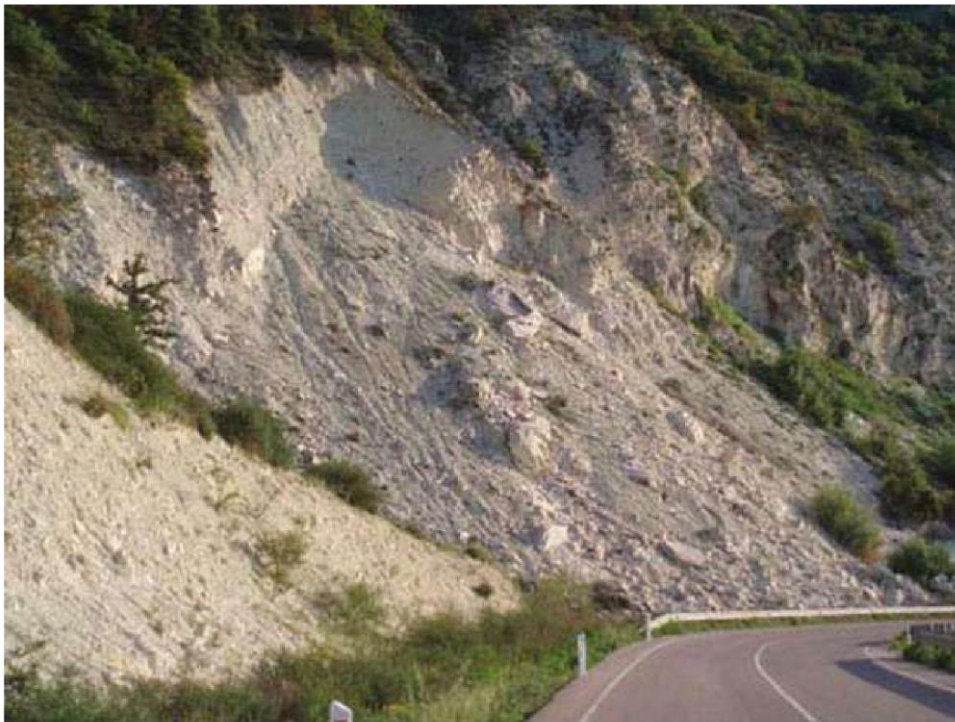
Fig. 1 Landslide, Paphos-Limassol Highway in Cyprus
