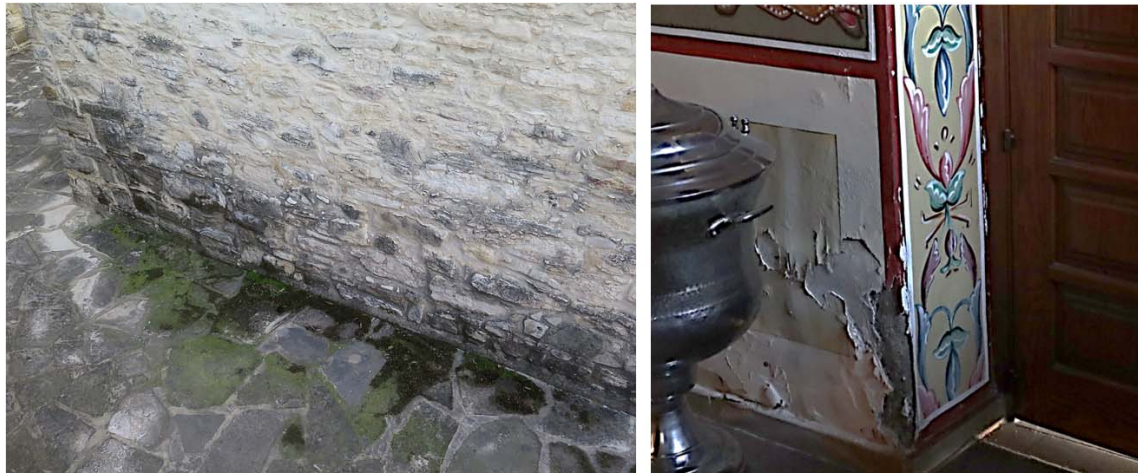
Figure 1: Left: Moss resulting from moisture; Right: Moisture damage to the corresponding area within the church
