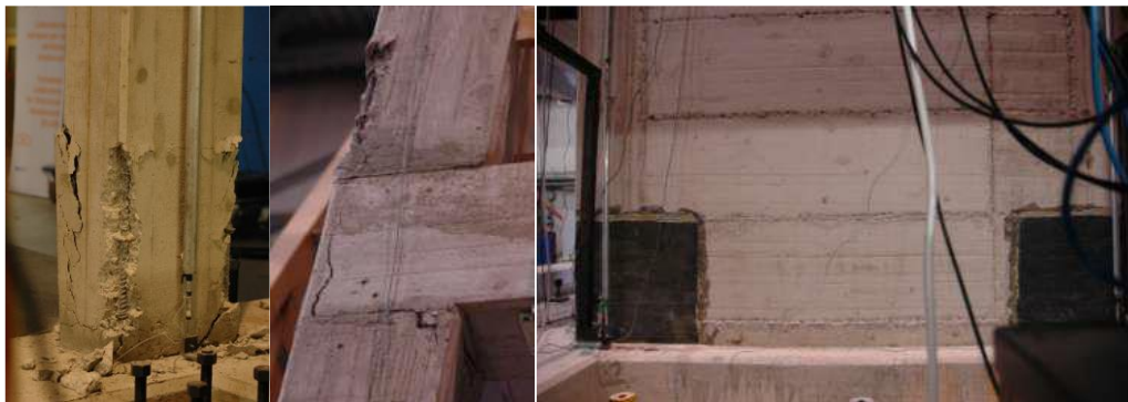
Figure 3.12: Lap-splice failure due to tensile forces appeared in the outer column on the east side of the south frame (left picture), lap-splice failure due to tensile forces appeared in the outer column on the west side of the south frame (middle picture) and hairline cracks that developed in the south wall (right picture) (Poljansek et al. , 2014)
