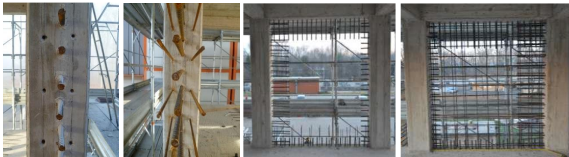
Figure 3.4: First connection detail of the new infill wall to the bounding frame with starter bars and short dowels (Dowels, dowels and starter bars, dowels and starter bars, dowels starter bars and web reinforcement)
