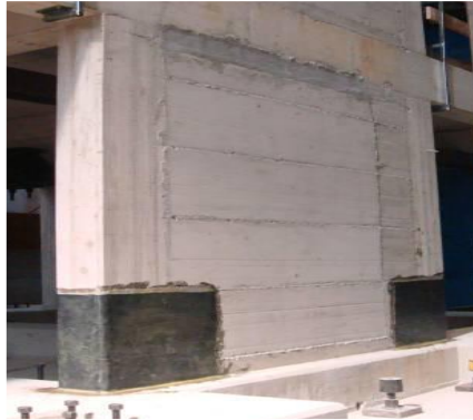
Figure 3.7: First and second connection details of the new infill south wall to the bounding frame
