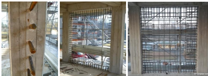
Figure 3.5: Second connection detail of the new infill wall to the bounding frame with only longer dowels (Dowels, dowels, dowels, and web reinforcement)
