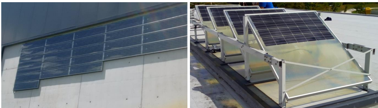
Figure 8: detail of ventilated façade on INGRID building during installation (left) and skylight (right)
